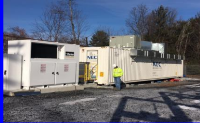
Dec. 2016, 2MWh Storage, 3MW PC
